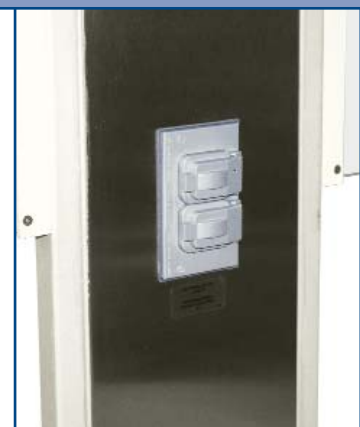
Interior duplex outlet
