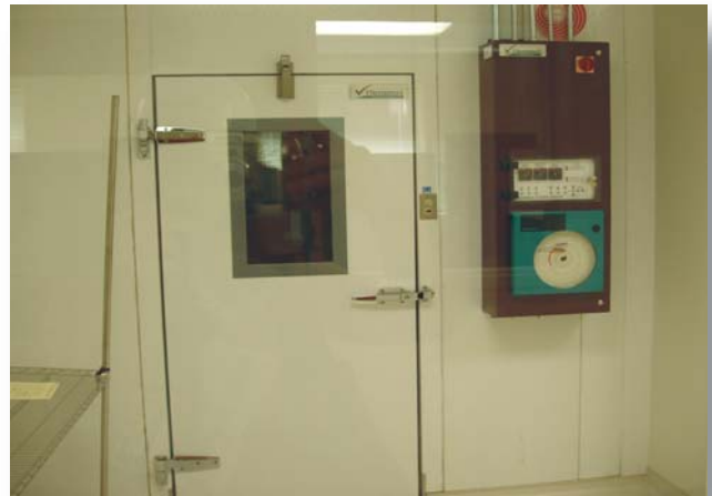
Walk In Cold Room
