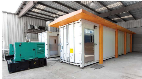
40' ISO Container BSL-3 Laboratory Building
